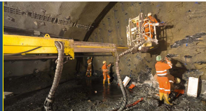
Since July 2006 the second tunnel of the Tauern Tunnel has been under construction on the A10 Tauern motorway. The project, worth EUR 109 m, is expected to be completed by May 2010.
