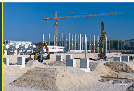
For the OMV gas compression station project in Lower Austria 10,000 m 2 asphalt was laid and 600 m 3 concrete foundation was manufactured. Planned completion is October 2008.
