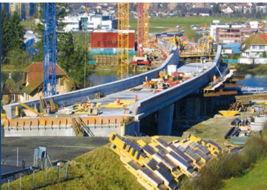
The Aar Bridge/Solothurn in Switzerland is planned as a continuous beam bridge with floating suspension and a total length of 387.36 m. It will be finished in 2008.
